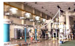
New Makkah West 380kV Substation
