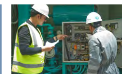
Dawadmi 380/132kV BSP Substation
