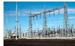
New Kandarah 380kV Substation
