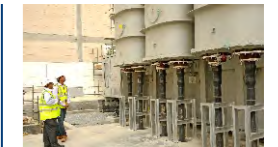
Al-Kudmi Project 380kV
