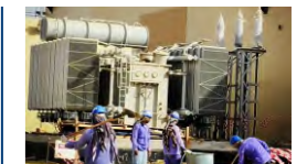
Shaybha NGL Power Generation Project Packages(1,2,3 & 4) (13.8, 230kV)
